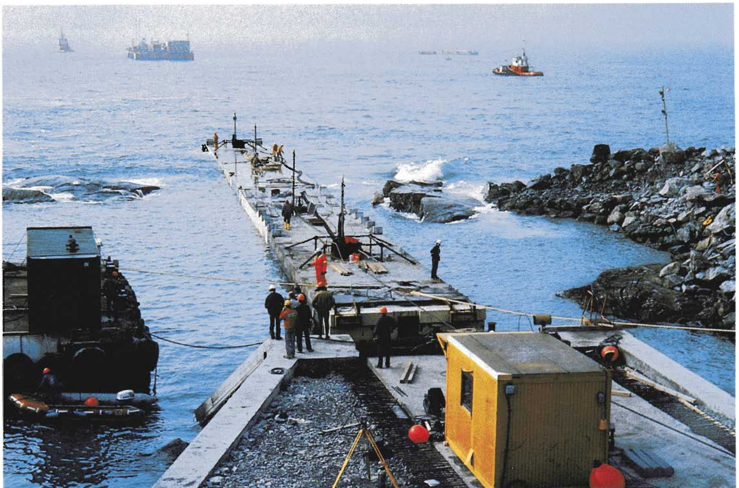
Landing of a pipeline in Western Norway involved the installation of a precast concrete tunnel here being installed.
